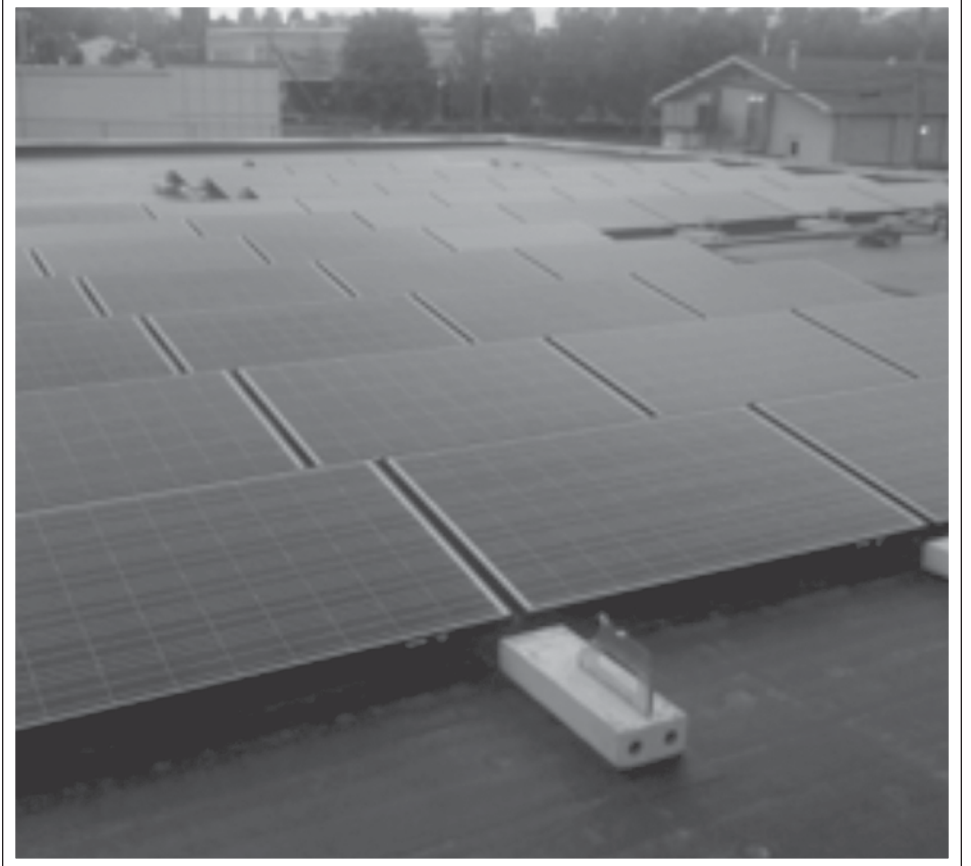
Solar panels on the roof of the Amity Teen Center
