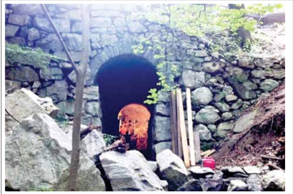
Peering into the western portal of the tunnel, an eerie orange glow envelopes the crew at work repairing the wall.
