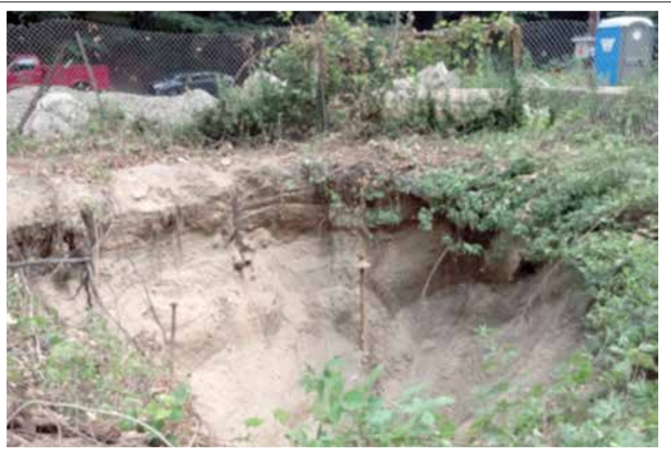
The cave-in area with sand eroded to a depth of 15 feet; exposed metal rods may have braced the old trestle timbers.
