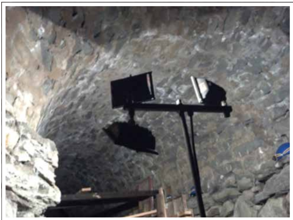
Rubble-stone sidewalls support the barrel-vaulted ceiling which is amazingly intact after 130 years.
