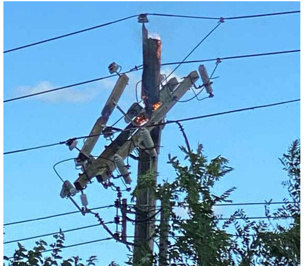
Electrical Fire on Pole
