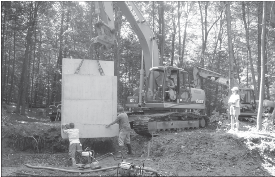
As Selectwoman Judy Williams watches, workmen from T.M. Wright Excavation are busy putting in abutments and footings for the construction of the bridge in the Wepawaug Conservation Area on September 22nd. The Orange Highway Department also had a representative there to help, Ken Ciola.
